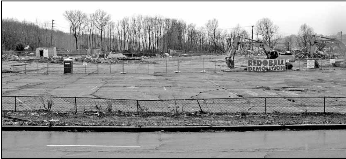
The old Grand Union, along with other stores, was demolished Mid-March 2006. Although Wood-Ridge officials have been planning redevelopment for years, the project was held up by a legal battle over the 5.7 acre property owned by Abe Oster. Mr. Oster attempted to develop his property by himself and resisted borough officials' attempts to condemn it for $3 million. The property was assessed at $4.5 million. Mr. Oster passed away in July 2005 and a settlement was reached with Oster's son, Avi. The property is crucial to the development because it provides access to Passaic Avenue.
