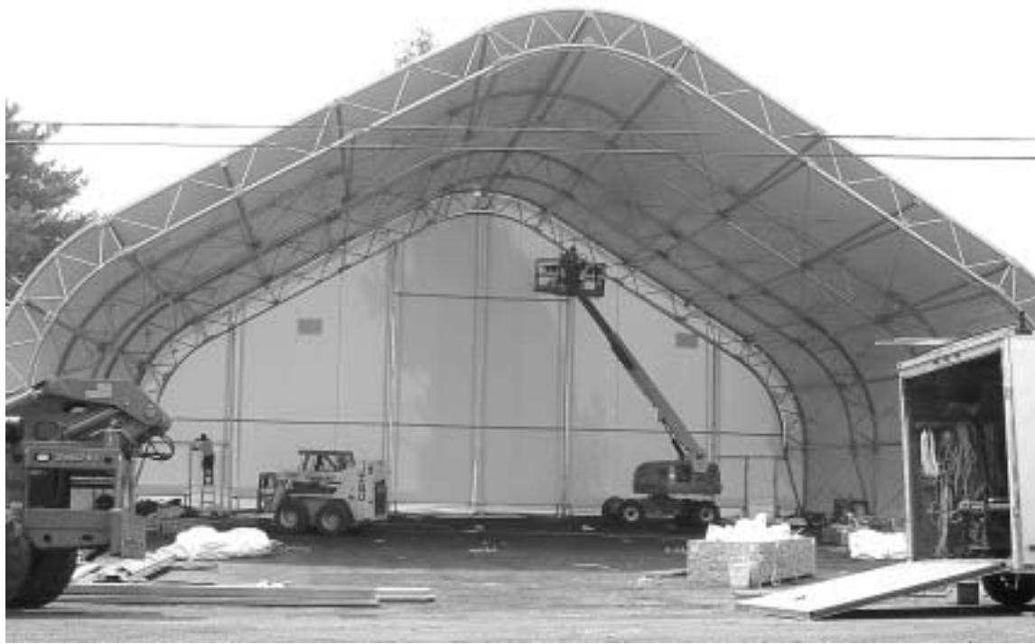
Construction photo taken August 15, 2002. When completed the structure held (l-r) Rescue Truck, Engine #1, Ladder Truck, Engine #2 and two Ambulances parked behind each other. Firemen's equipment was set along the back. A trailer behind the unit held the Department's offices. Old Engine #1 was parked by the trailer.
