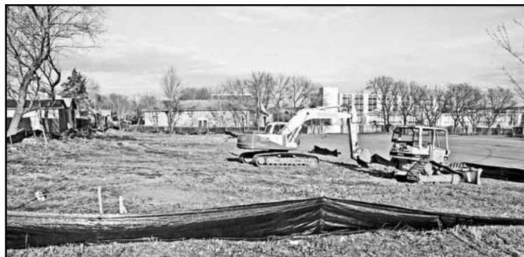
This land was sold by the Borough in June 2006 for $1.73 million with the funds slated toward the cost of the Depken Field upgrade. View from Oldfield & Washington, facing north.
